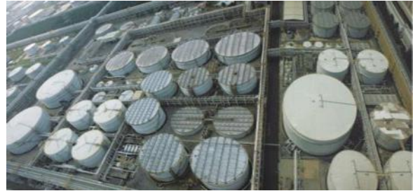
Wastewater Treatment Plant (After improvement)
