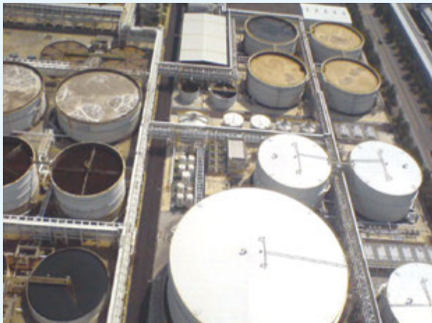
Wastewater Treatment Plant (Before improvement)
